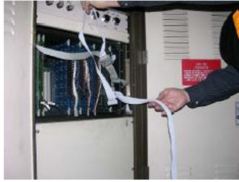
Flat Cable splice to new CPU board
