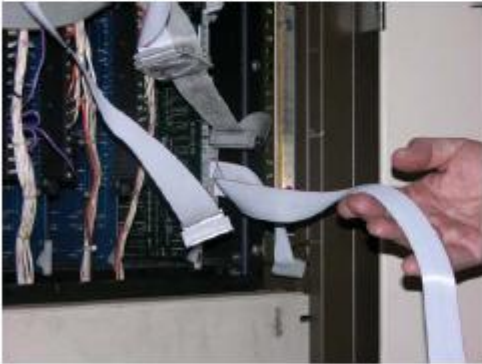
Flat Cable to PC from aux communication board
